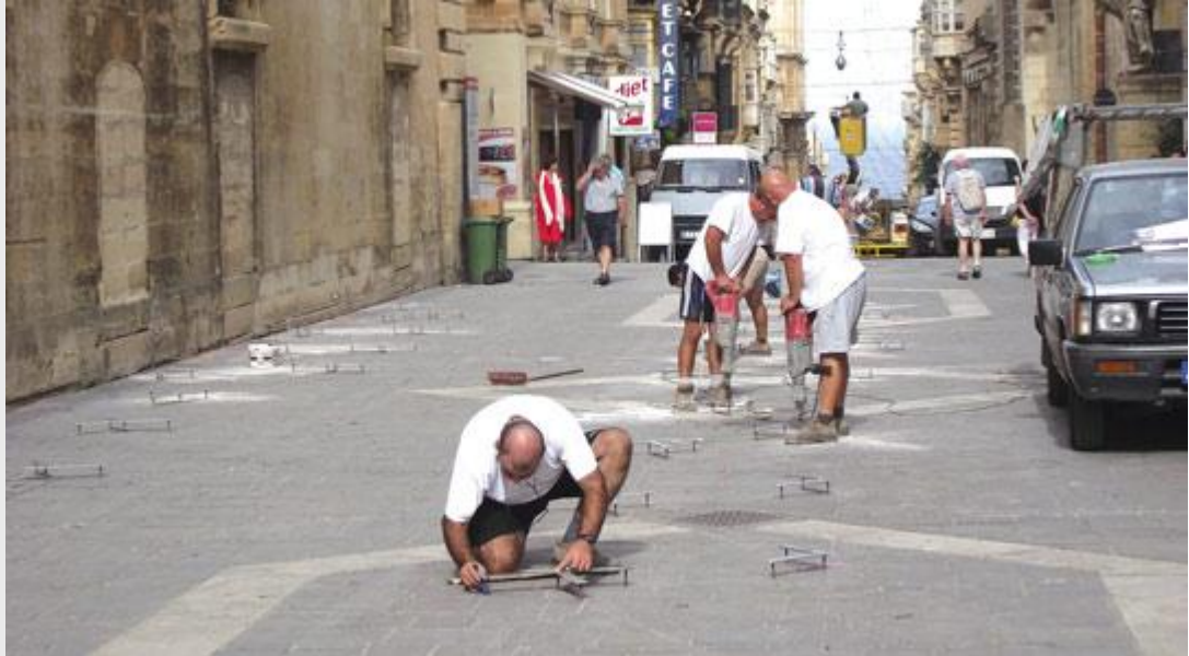
Workers fixing metal plates marking parking bays for Members of Parliament, in that part of Merchants Street that is taken up by the open-air market during weekday mornings. Photo: Jason Borg
