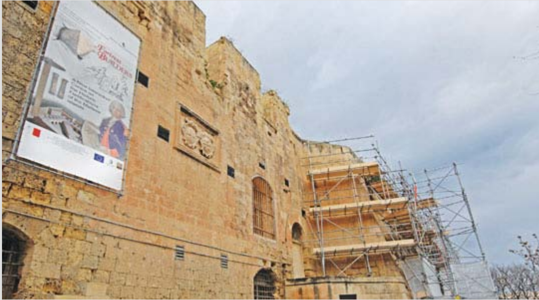
Scaffolding has been put up near Biago Steps for restoration works to be done. Photo: Jason Borg.
