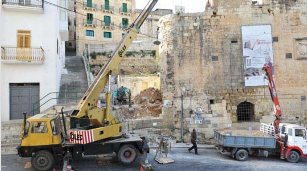
Biagio Steps will be restored to be used as an interactive centre that will focus on Malta's fortifications. Photo: Chris Sant Fournier
