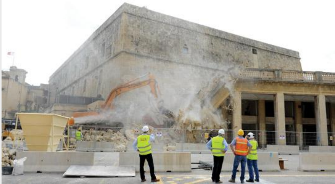
The demolition of the arcades next to St James Cavalier at Freedom Square, Valletta, forming part of the City Gate project continued yesterday. Photo: Matthew Mirabelli
