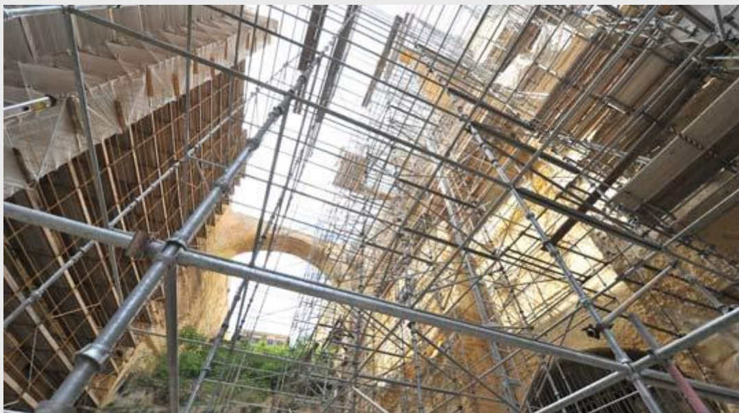
A string of bastions in various cities including Valletta are being restored at a cost of €36 million. Picture shows the maze of scaffolding by the bastion rising up from the ditch below the Upper Barrakka Gardens, Valletta. Photo: Jason Borg
